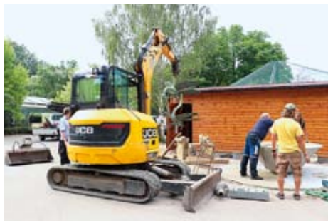
Instalace fontány se sovkpturou váček. KM Installation of the fountain with a dragonfly sculpture
