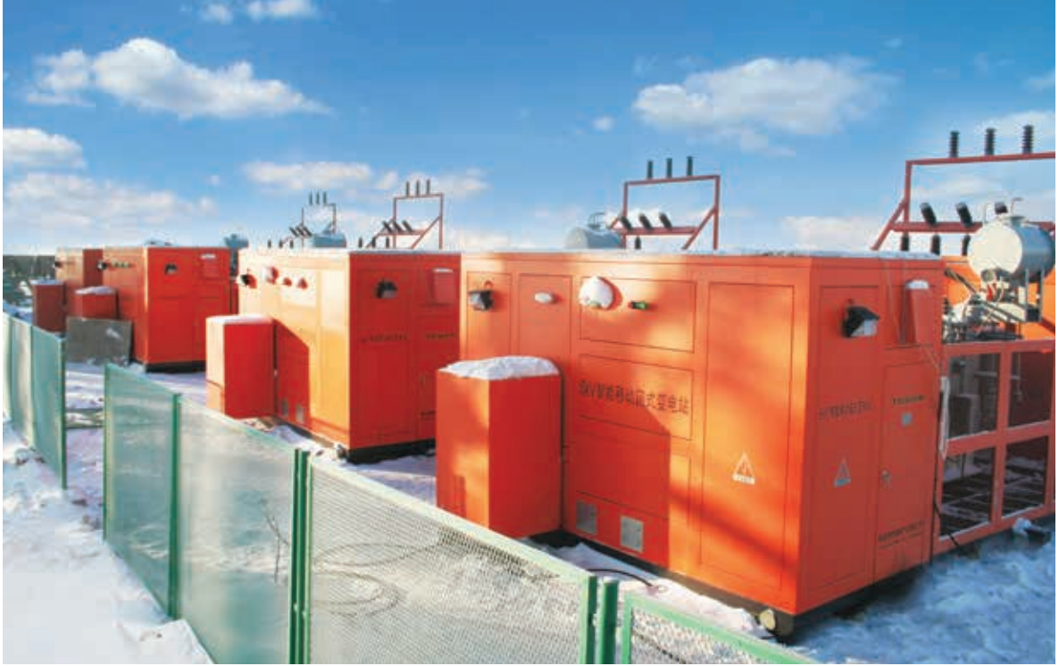
40.5kV Skid Mounted Substations at Open Pit Coal Mine
