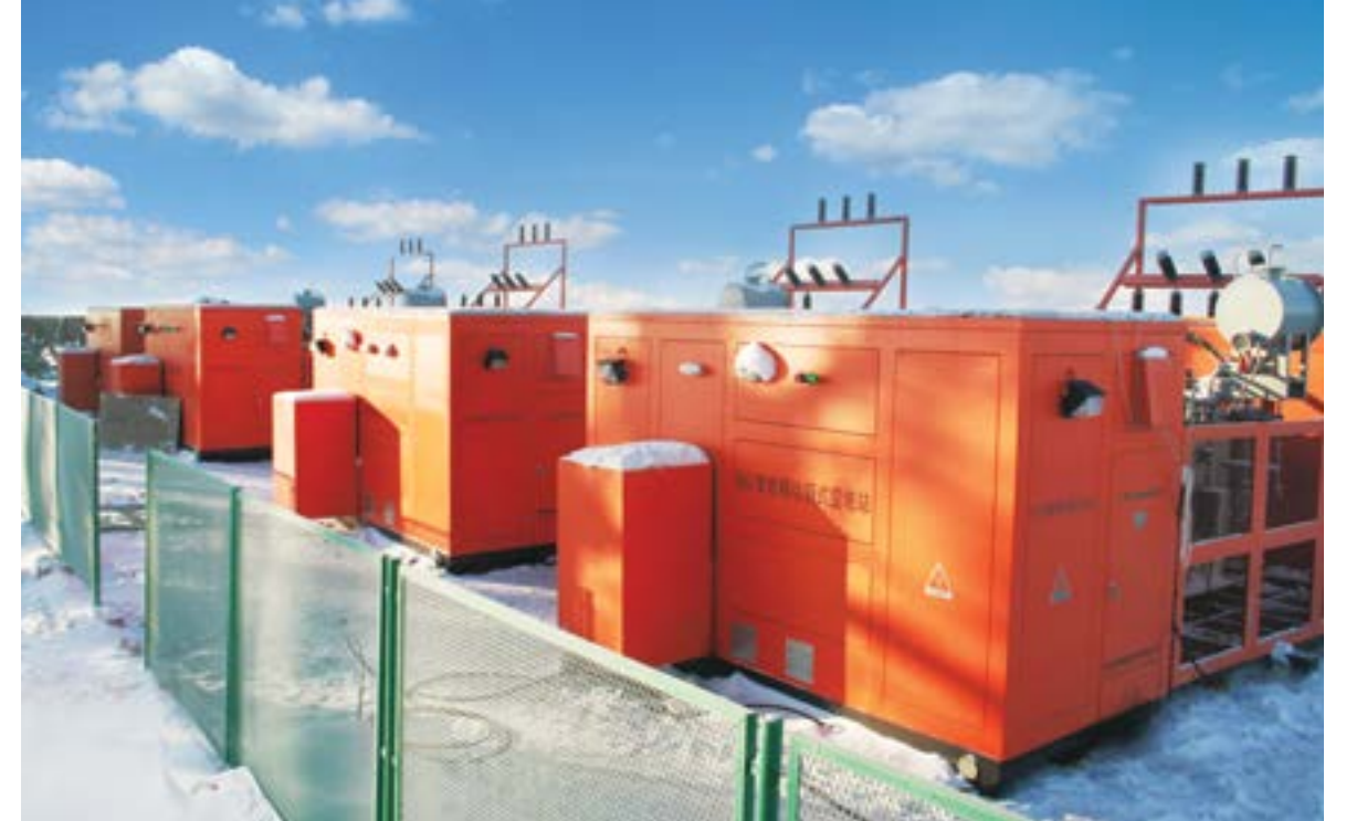
40.5kV Skid Mounted Substations at Open Pit Coal Mine
